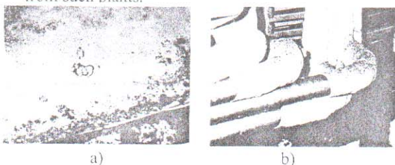
Fig.1. Slime in the transformer (a – inside the tank, b – on windings)
