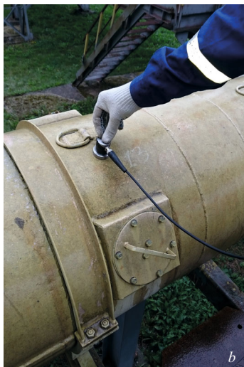
Fig. 7. PD location using electromagnetic ( a ) and acoustic ( b ) sensors during diagnostic examination of isolated bus ducts.
